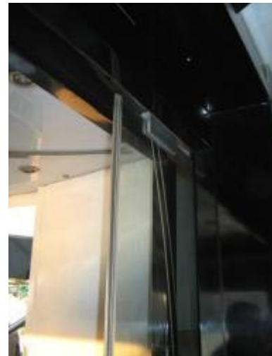
Picture 38 provided a break using rubber to reduce shock and friction resulting in cracking door leaf
